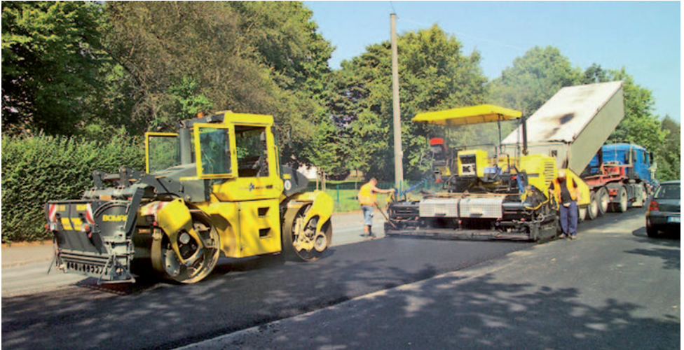
Fig. 7 Laying and compacting with the BOMAG BF 600 P and the BOMAG BW 174 AD-AM
