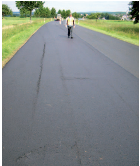
Fig. 80 Transverse and longitudinal cracks cause by the use of a too heavy roller
