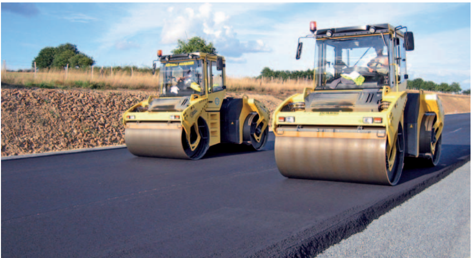
Fig. 51 BW 203 AD on a 16cm asphalt bearing course with a compaction performance of 250 t/h
