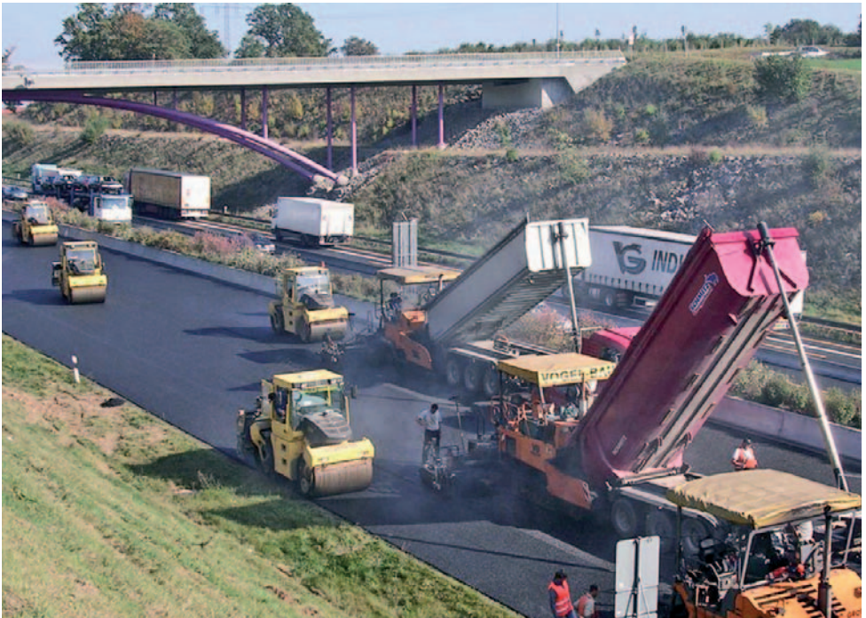
Fig. 47 Laying and compacting an asphalt layer using three finishers and five vibratory rollers (10t). Laying width > 10m; daily output > 3.000t.
